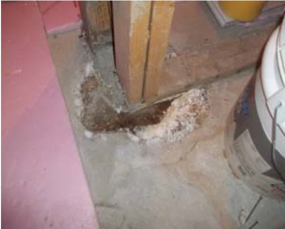
Efflorescence noted. Monitor for further staining and or damages.
